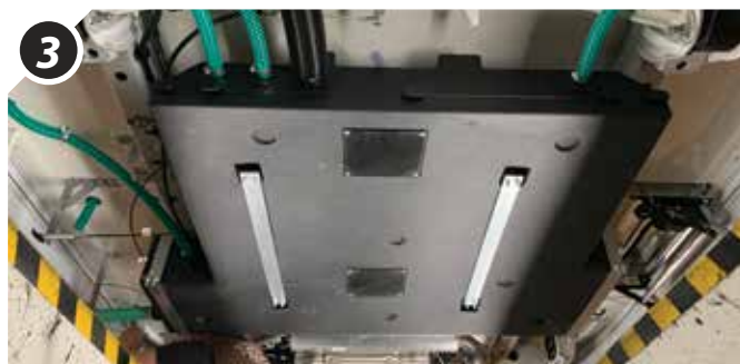
Insulation for grey water tanks
